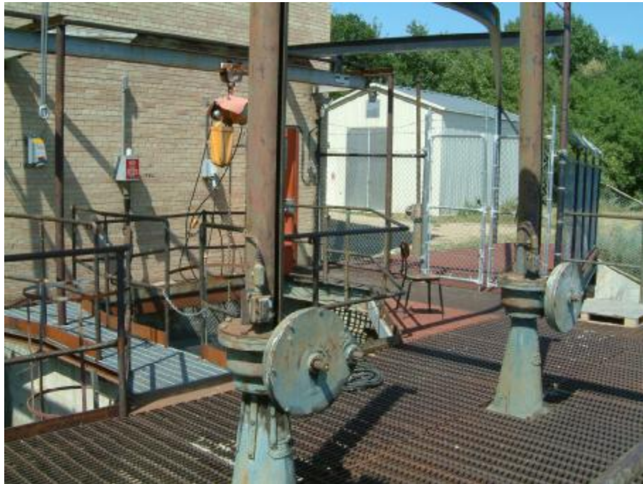
Figure 4-3 QE Low Lift Manual Gates
