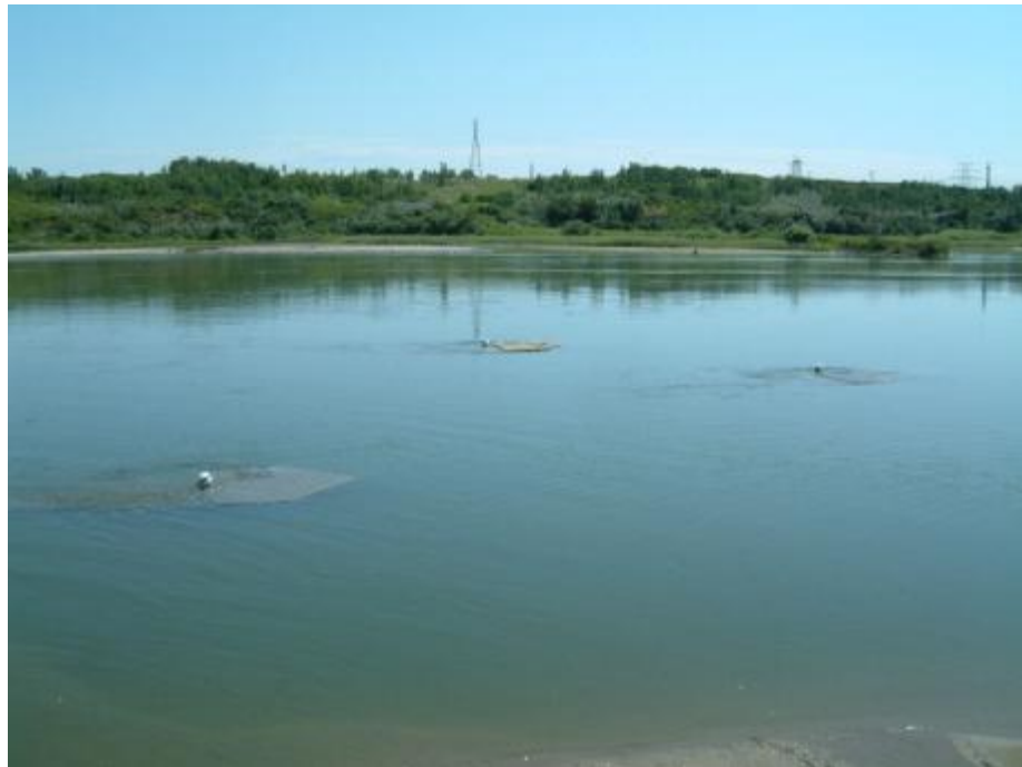
Figure 4-2 QE Low Lift Intake Structures
