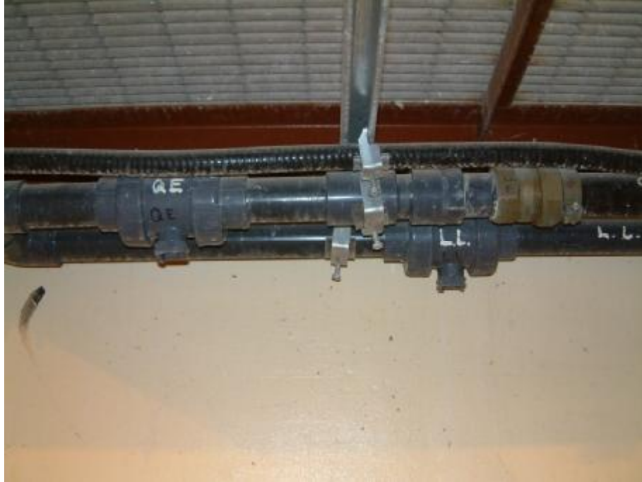
Figure 4-11 Potassium Permanganate Feed Point Selector Valving in Chemical Feed Building
