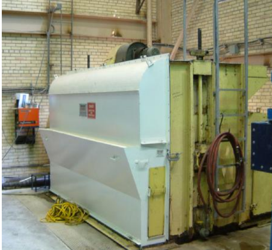
Figure 4-4 QE Low Lift Traveling Screen
