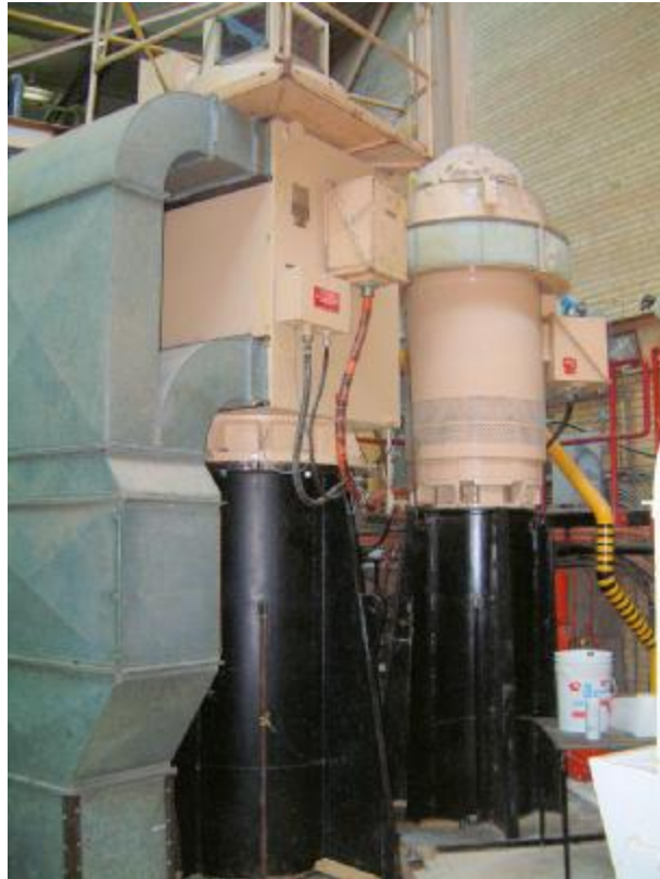
Figure 4-1 A QE Low Lift Pump
